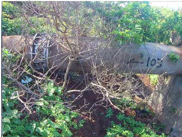
Coupling 103 (south side)
