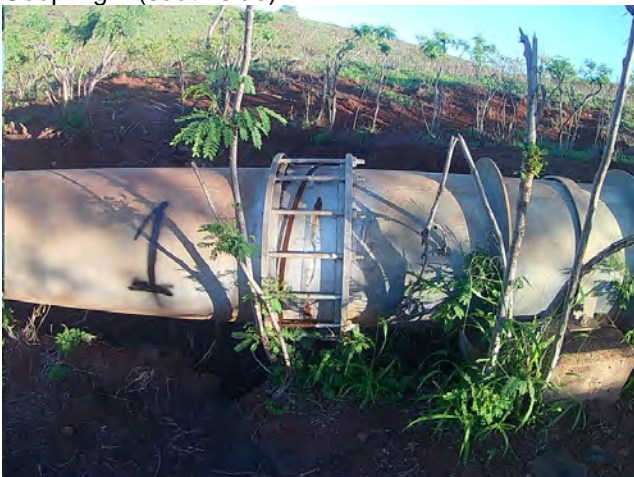
Coupling 1 (south side)
